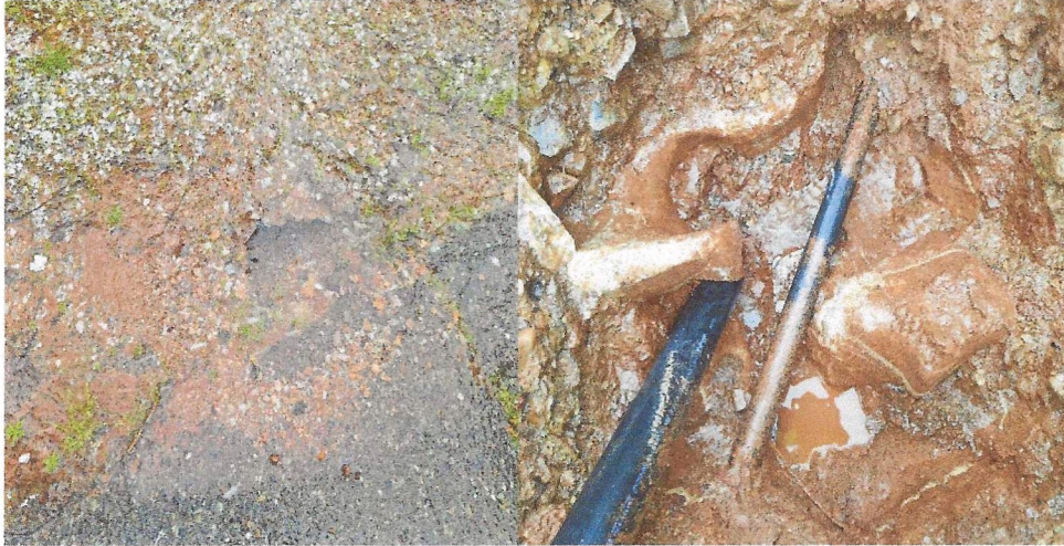
50 GALLON PER MINUET LEAK
